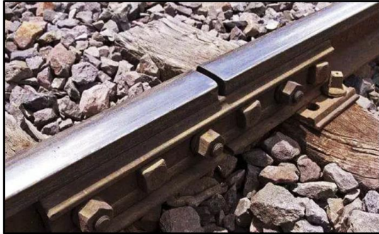
gaps in railway tracks
