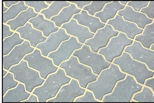
gaps in pavement
