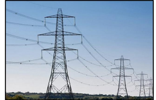
sagging overhead electric wires
