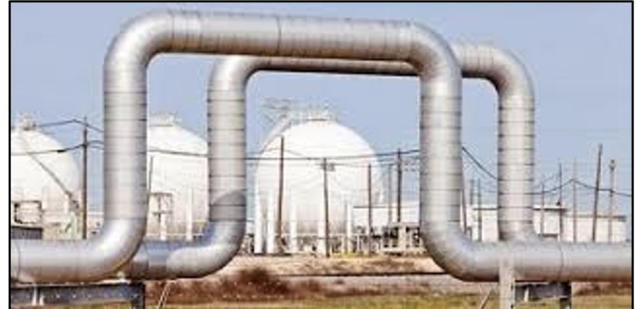
loops in pipes
