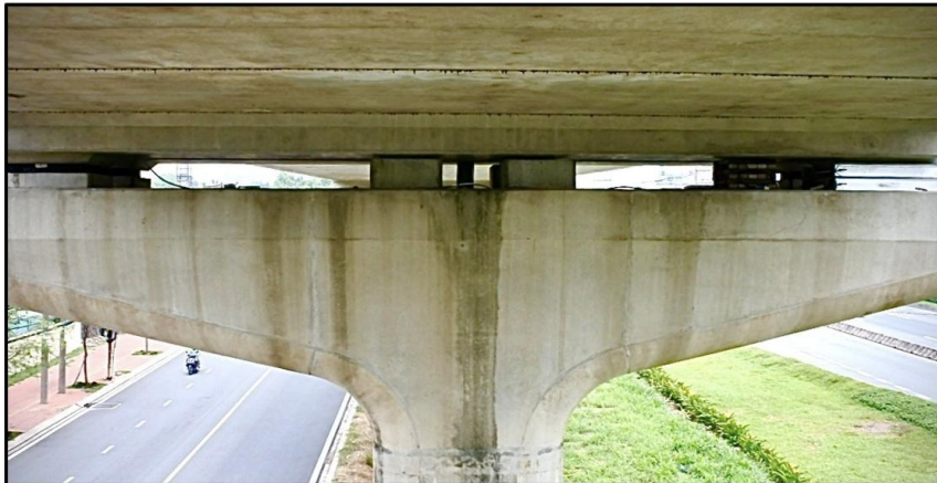
rollers in bridges
